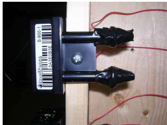
Figure 33: Terminals with electrical tape
