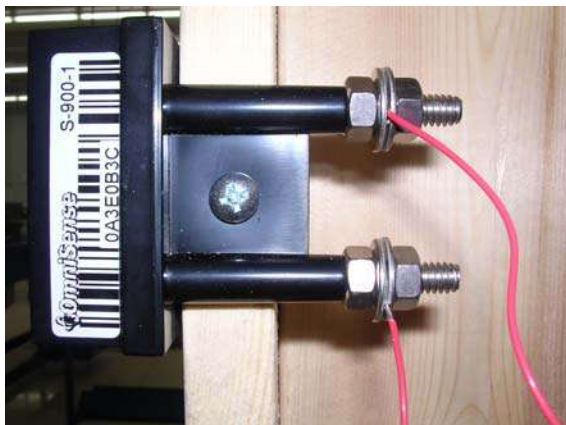
Figure 32: Sensor wires connected
